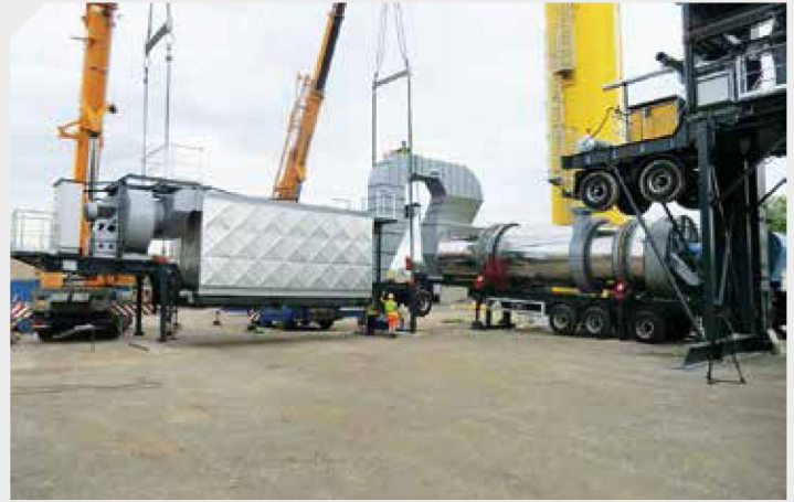
// DUST COLLECTION SYSTEM
