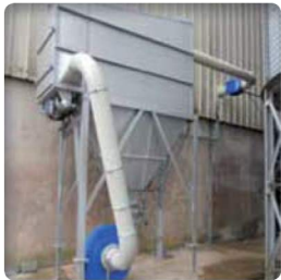
Under a dust collector
