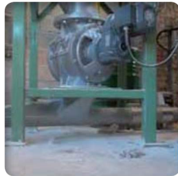
Feeding a pneumatic conveying pipeline
