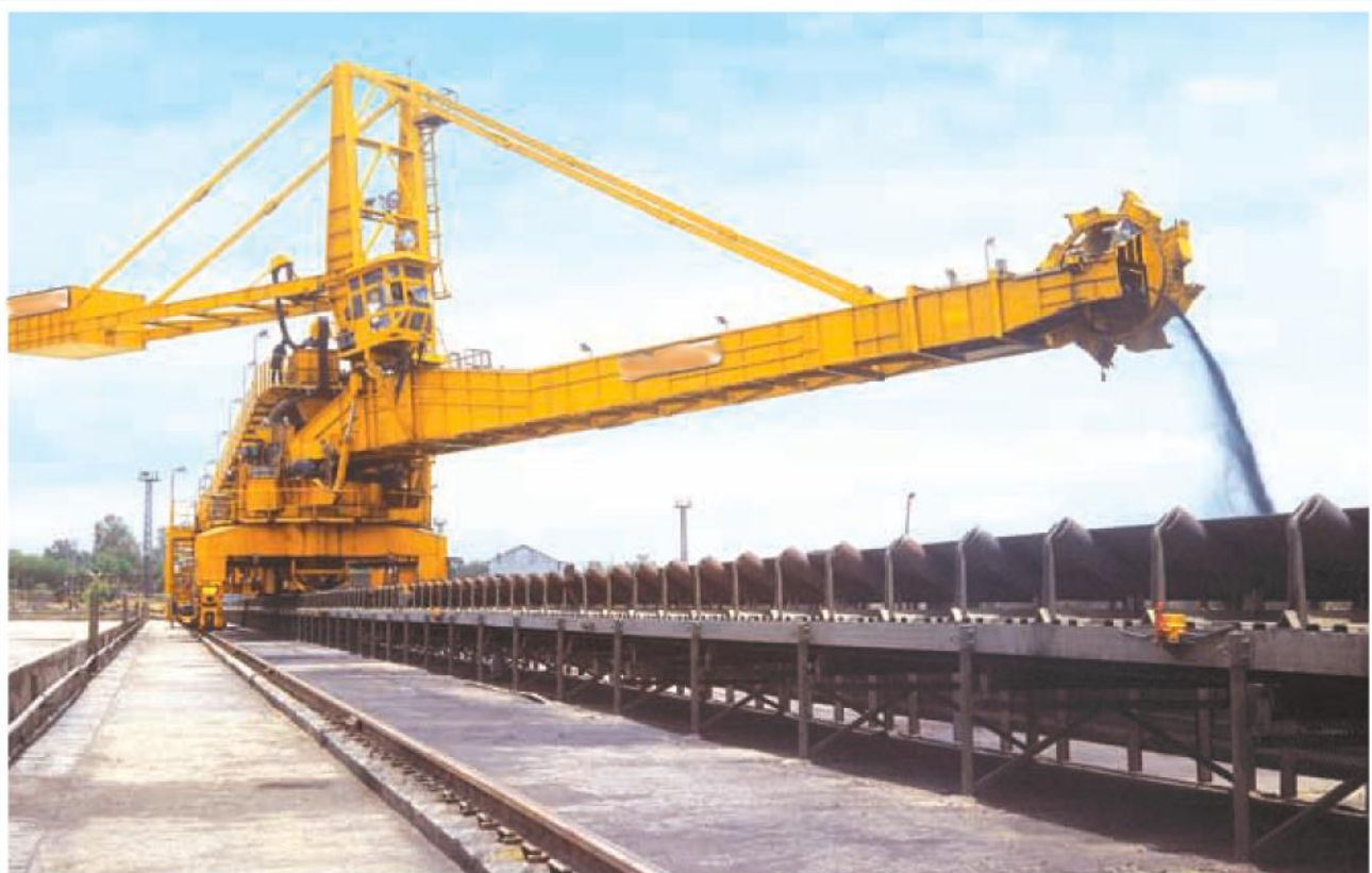
Stacker-Cum-Reclaimer in Operation at Thermal Power Station of Maharashtra State Electricity Board
